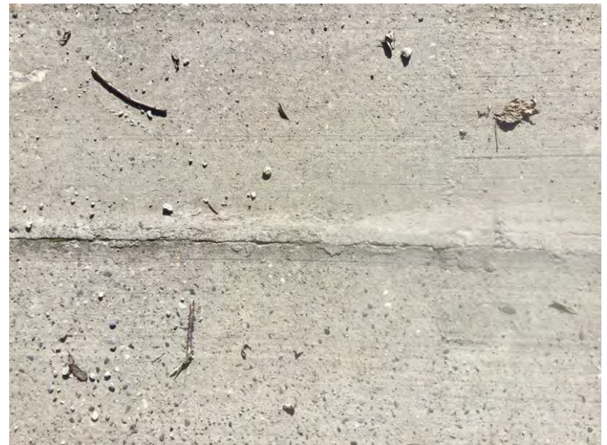
Hairline cracks noted at surface in all deck joints
